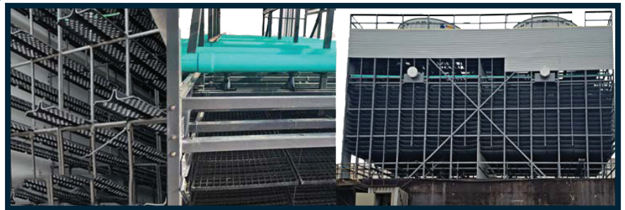
SPLASH TYPE COUNTER FLOW COOLING TOWER
